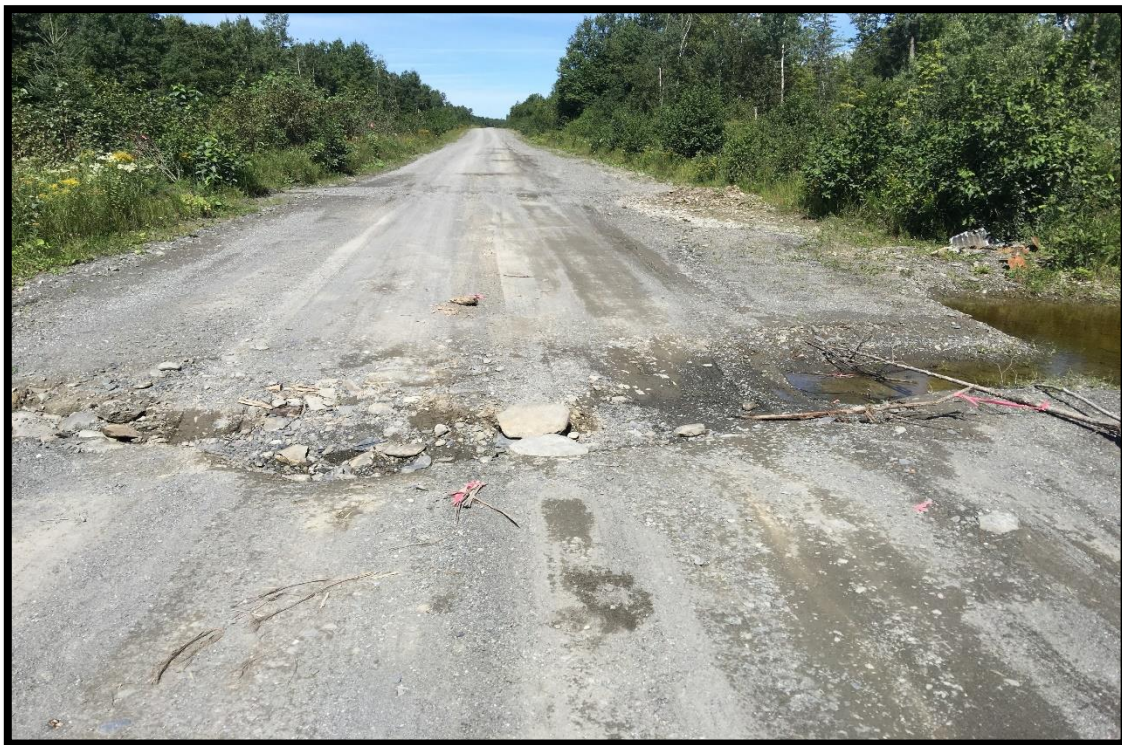
Figure 19 Photograph showing road issues that could make a site inaccessible
