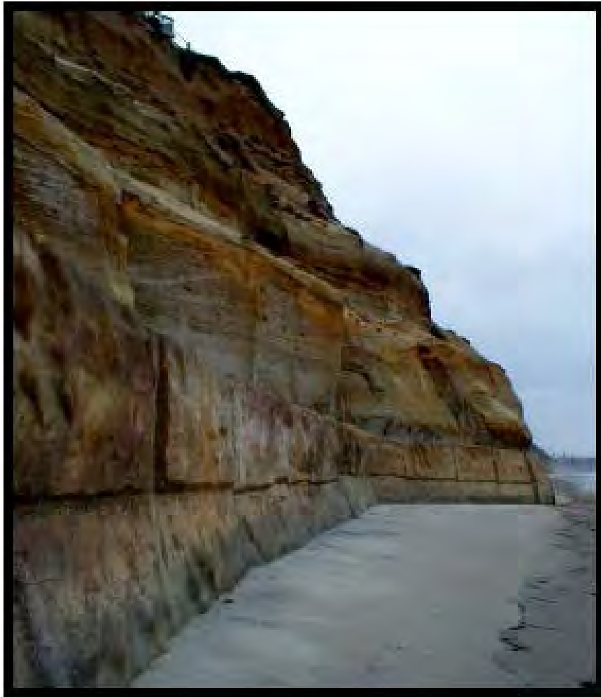
Figure 2 A seawall in Encinitas (California Department of Boating and Waterways and State Coastal Conservancy 2002)
