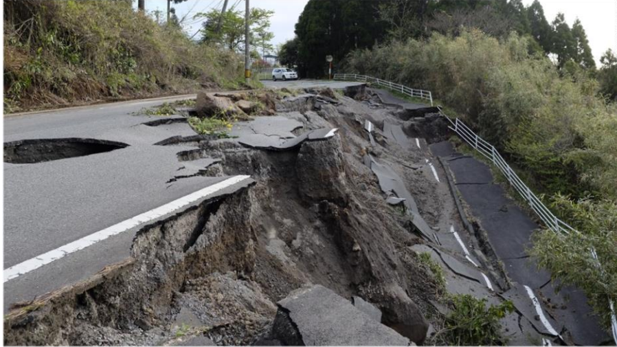
Figure 5. Road damage from the 2016 Japanese 7.0 earthquake
