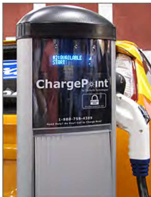
Figure 6 Level 2 Charging Station. Source: ChargePoint Network 2015
