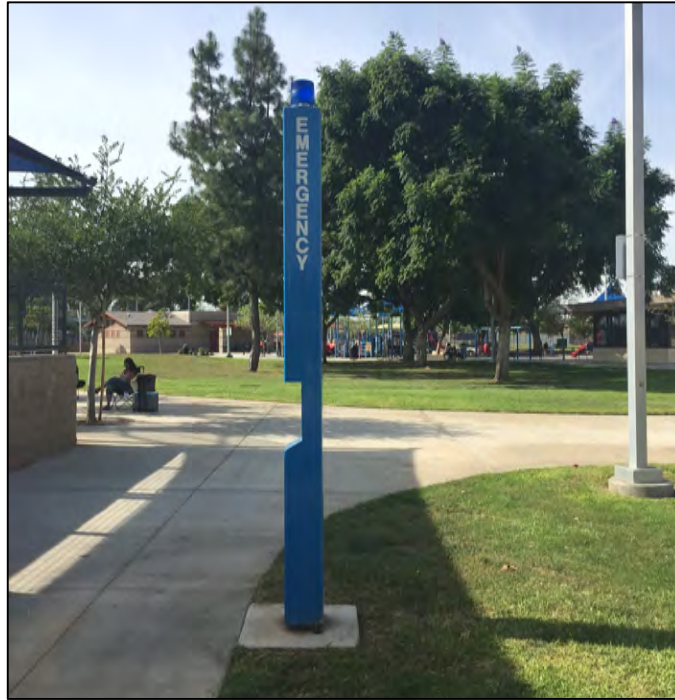
Figure 25 Emergency Call Boxes
