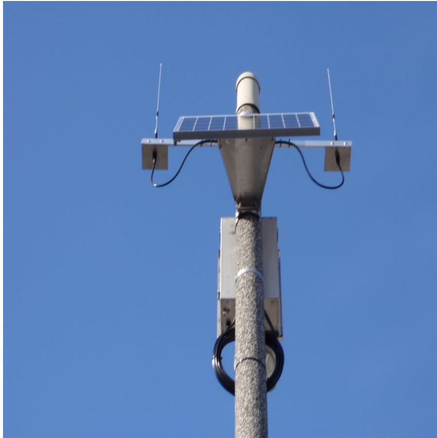
Figure 1: Smart grid DCU communications tower
