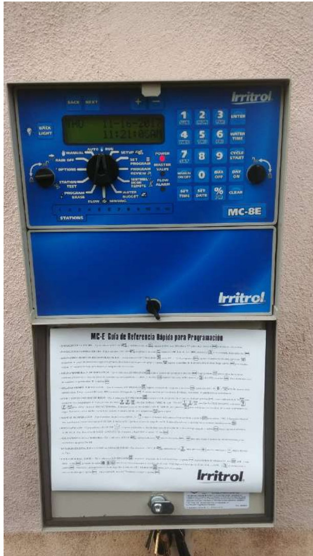
Figure 4: Field photo of controller D, a wall-mounted Irritrol box with up to 12 connections
