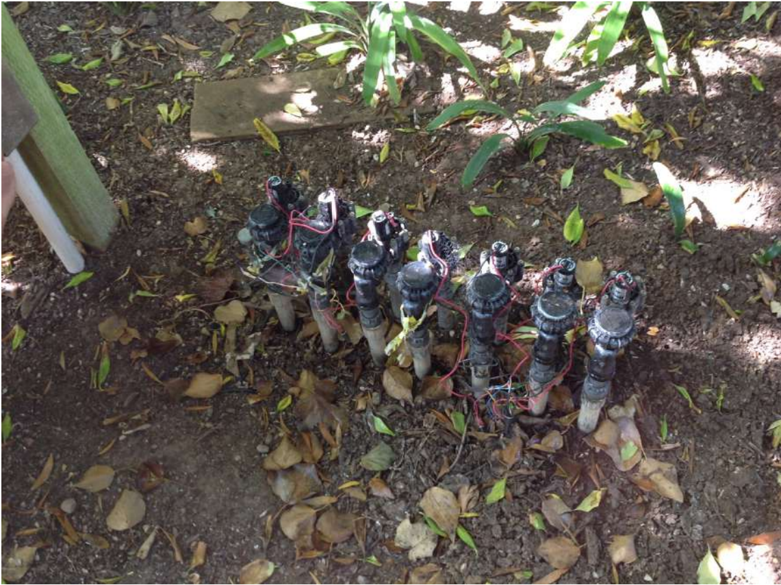
Figure 10: Dense line of above-ground control valves for Controller C
