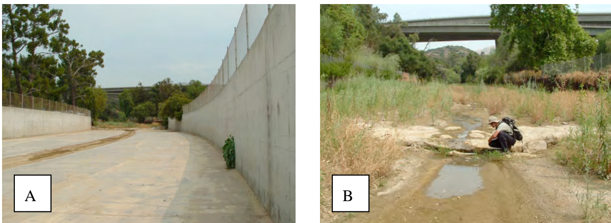
Figure 10. (A) Browns Canyon under the 118 freeway overpass; and (B) A hybrid portion of Browns Canyon where the natural creek channel becomes a concretized box channel
