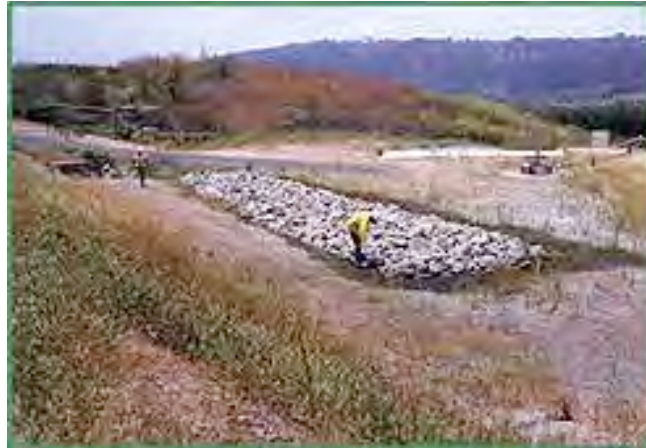
Figure 11. An extended infiltration basin that was constructed by Caltrans, San Diego County
